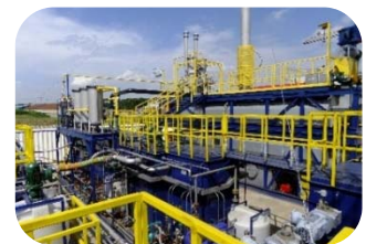
3 t/h Dual plant thermal desorption
